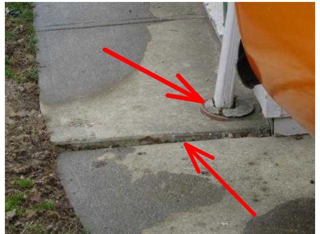
Trip hazard and downspout need to be resealed
