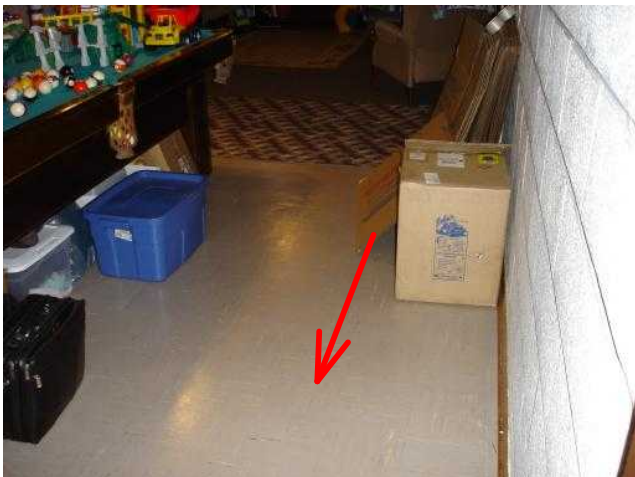
Possible Asbestos floor tiles
