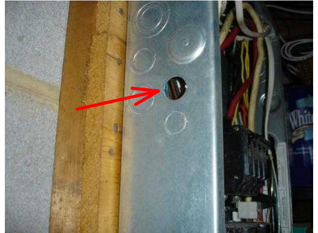
Knockout needs to be sealed
