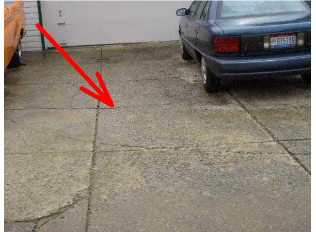
Concrete in driveway needs repaired
