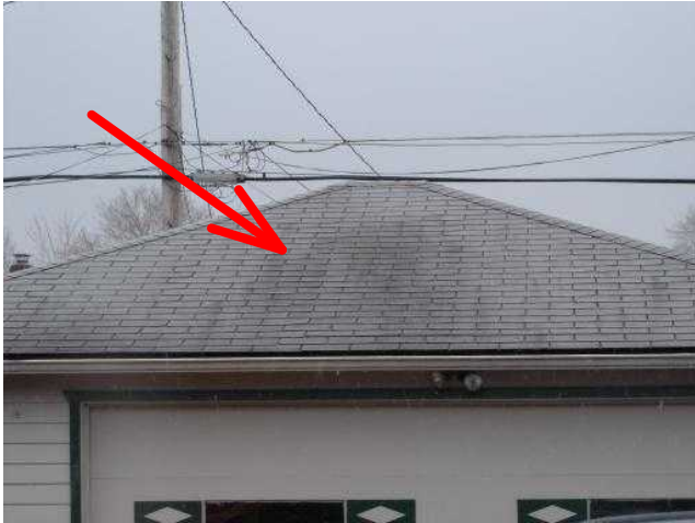
Curling and Cupping Shingles
